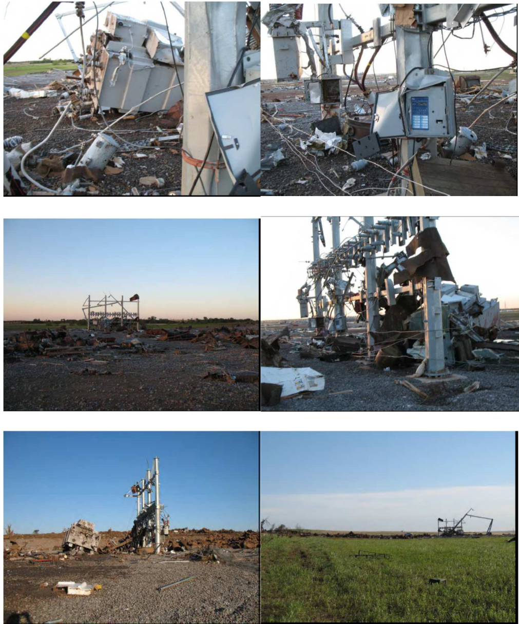
FIG 6. SUBSTATION DESTROYED BY TORNADO33
